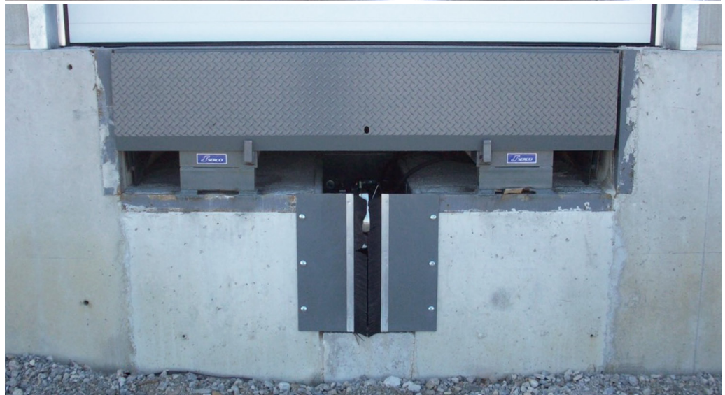
Fig.7 Loading Docks Concrete was poured to hold vehicle restraint and dock leveler.
